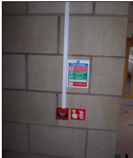
Typical fire call point
